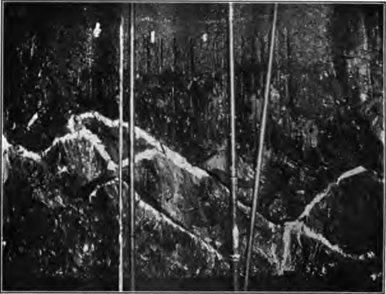
PLATE 2. SHOWING WATER BEARING CRACKS WHICH HAVE BEEN FILLED WITH GROUT. THE CLEAN-CUT SHARPLY DEFINED WHITE SEAMS SHOW THE EFFECT OF LETTING THE SAND OUT SO THAT THE SPACE IS FILLED WITH SOLID CEMENT. THE BLURRED, LESS DISTINCT SEAMS, HAVE FINE SAND MIXED WITH THE GROUT AND WHILE WATERTIGHT THE FILLING MATERIAL IS NOT SO HARD AS THE CLEAN GROUT.
